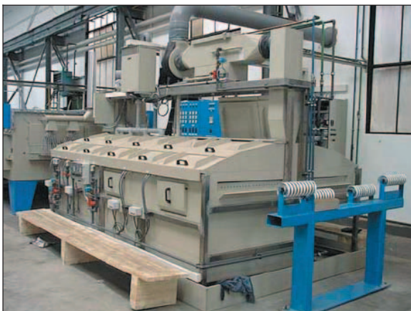
View of cleaning plant
