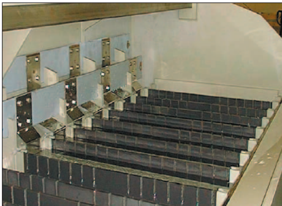
View of cleaning plant
